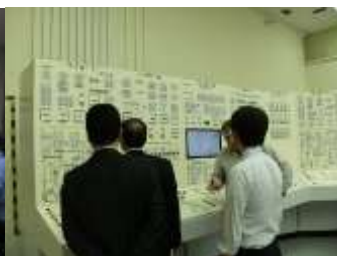
<Training Center at Novovoronezh NPP>
